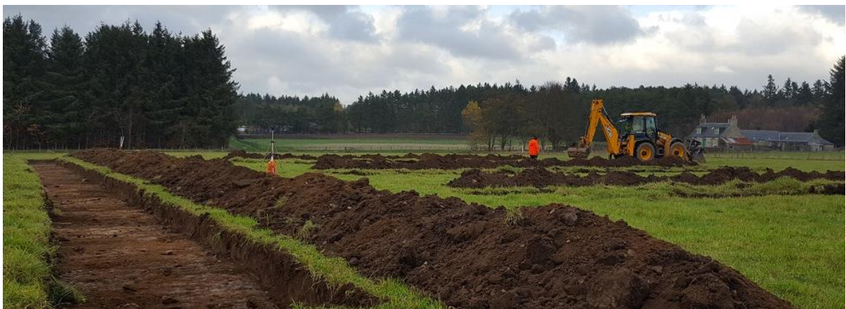
This photo helps to illustrate the number of trenches put in for the Stone Circle site
