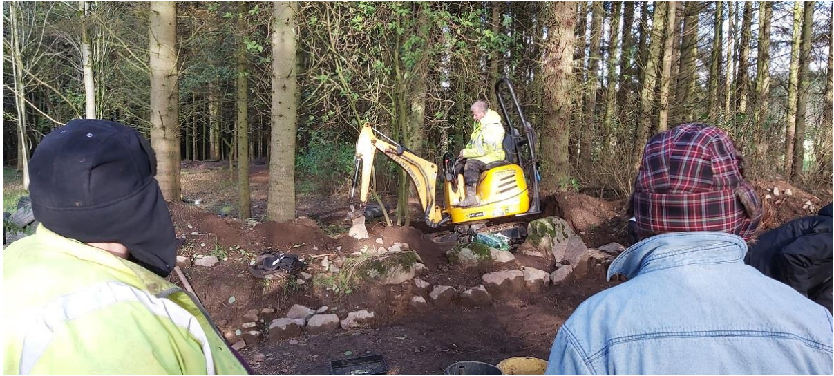
Robbie Cadger sets to work on leveling out the spoils heaps and surround ground
