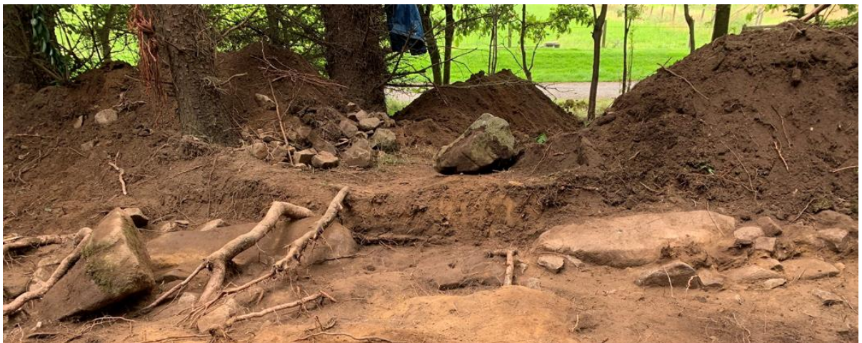
Roots removed but further cleaning required
